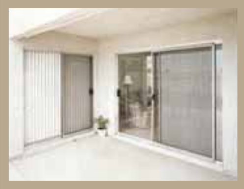
before: MILL FINISH ALUMINUM SLIDING DOOR
